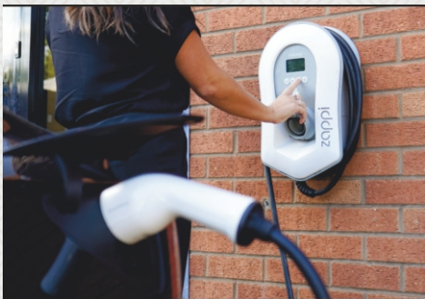
EV CHARGING POINT
